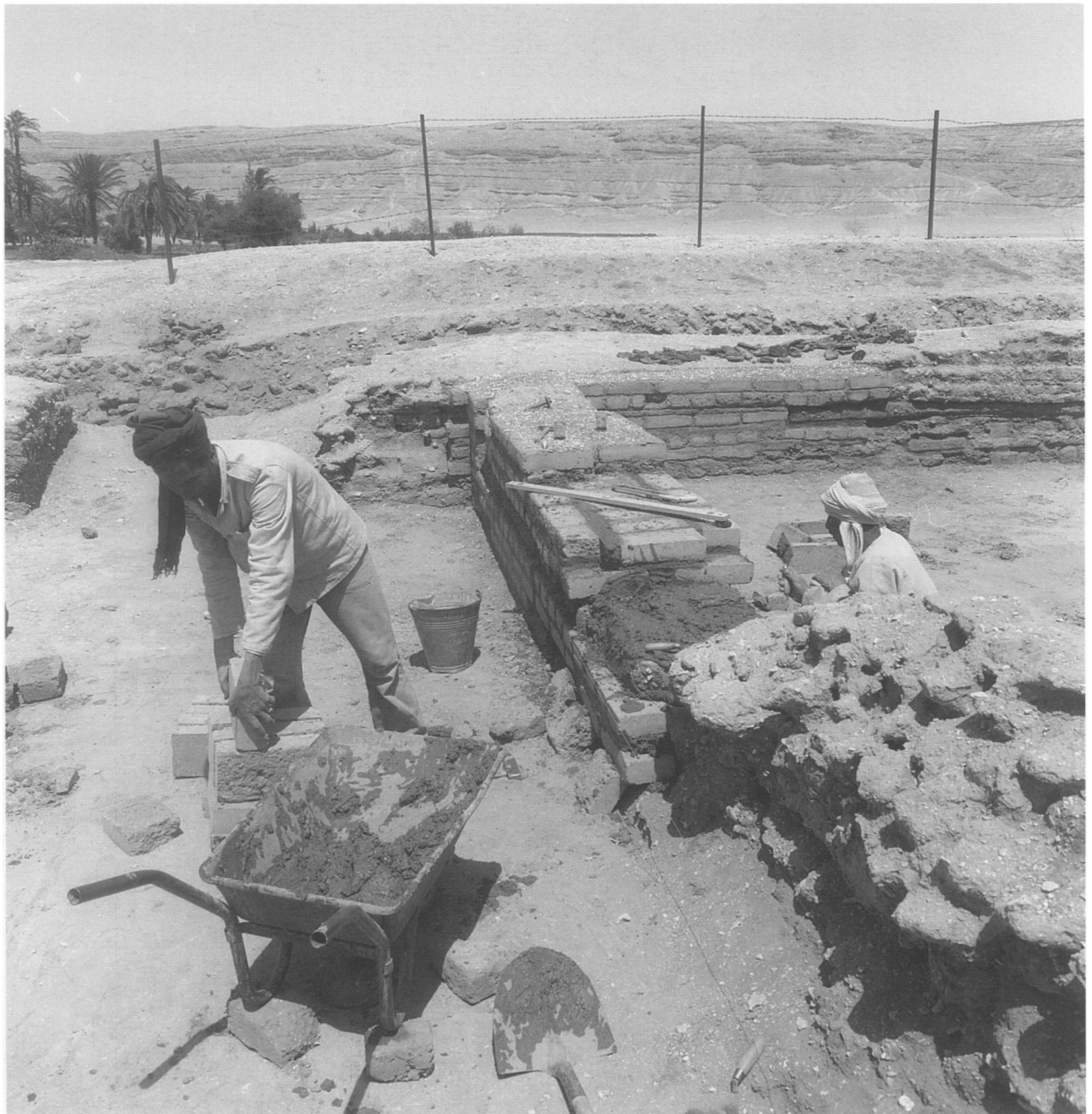
Conservation at the North Palace, showing a stage in replacing rotted bricks with new bricks
